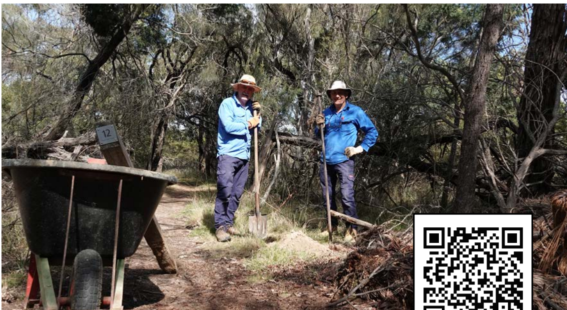
FOGMR members Terry and Pete replacing old posts on the Discovery Trail.
